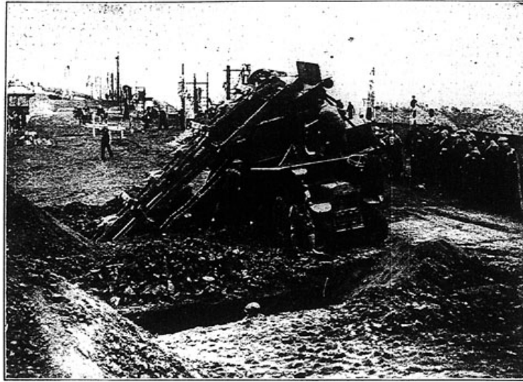
Figure 29.2: Trenches being made at the North Shore, Blackpool, with pneumatic drills and excavators. Manchester Guardian , 29 September 1938, p. 7.
